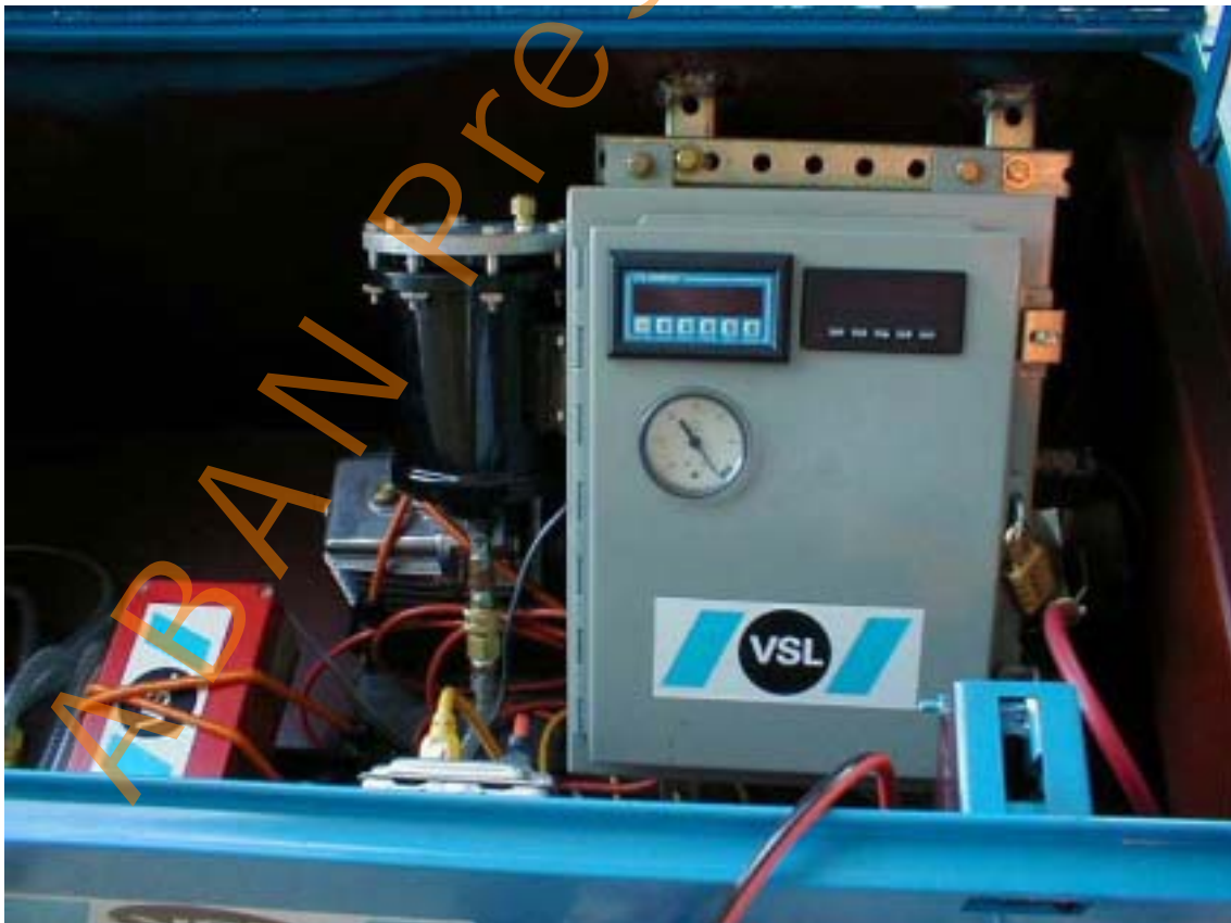
Fig. 21: Vacuum control and grouting equipment for tendons with defective grouting
